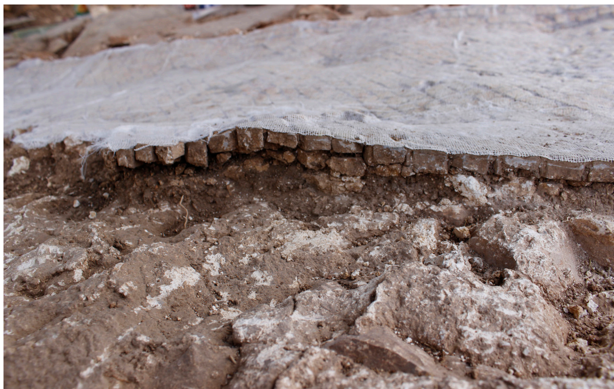
FIG. 9. The soil layer in between the bedding layer and nucleus in Room 3.
